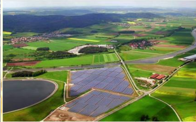
Muehlhausen, Bavaria, Germany, 6 MW SunPower T0 Tracker
